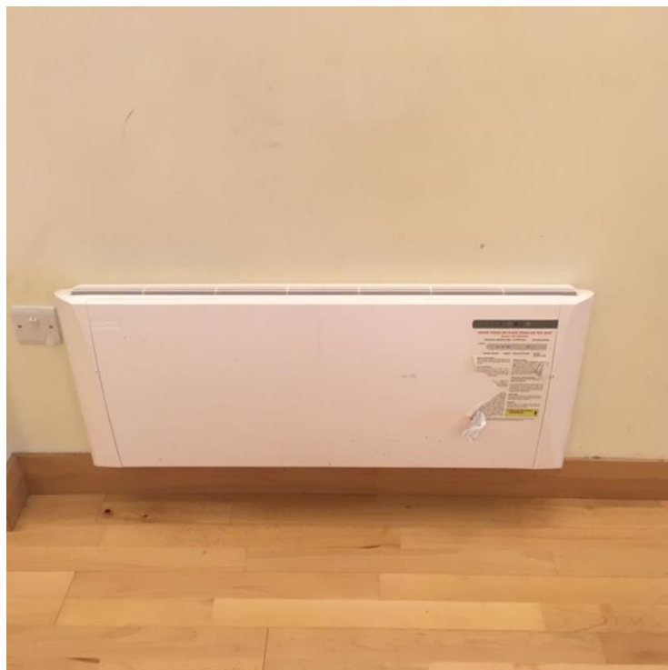
Figure A1.8 – Studio ground source heat pump – heating emitter
