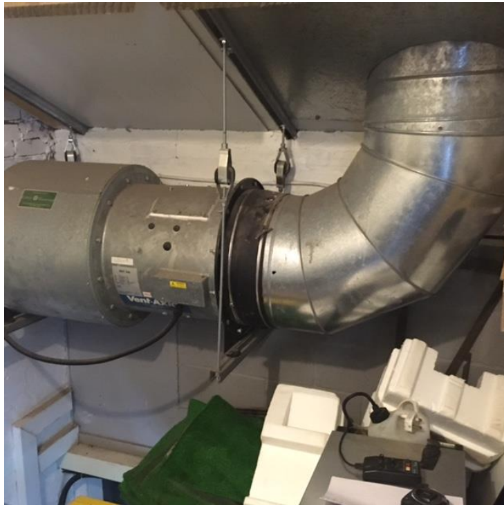
Figure A1.7 – Existing hall extract fan
