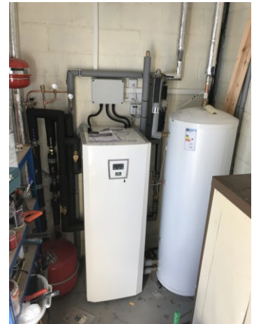
Heat pump system
